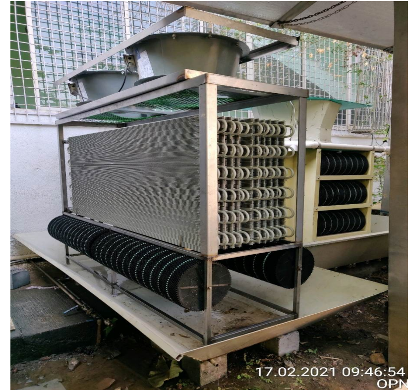
30 kW panel water heat exchanger
